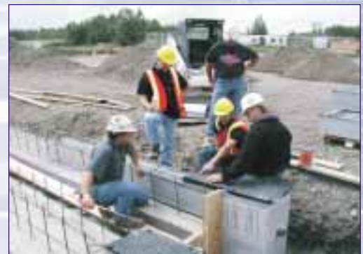
UTV composting plant in Canada - installation of aerating equipment by local contractors is supervised by UTV
